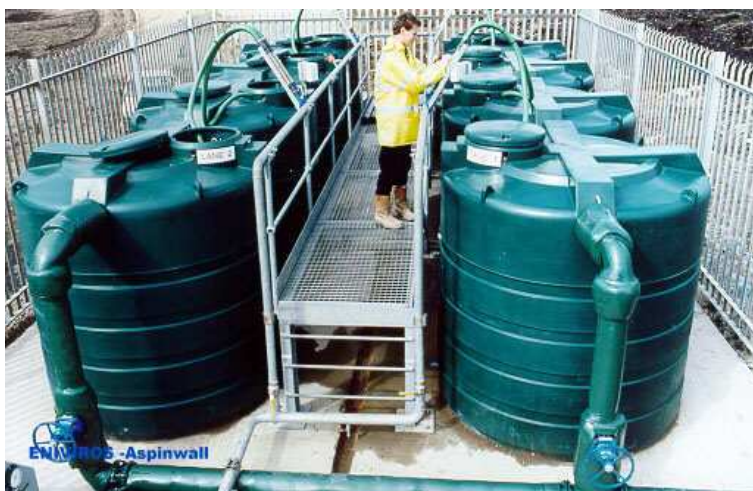
Figure 1. Methane stripping plant for Greater Manchester Waste Disposal Authority
