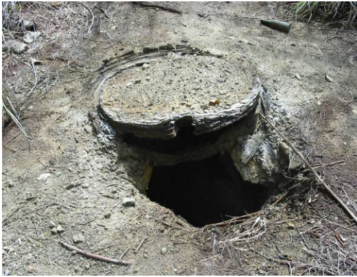
Sewer Manhole Corroded by Hydrogen Sulfide Gas, St. Croix
