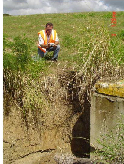
Hoyle, Tanner's Dick Perez Investigates Sinkhole by Sewer Manhole, St. Croix
