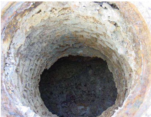
Manhole Concrete Deteriorated by Hydrogen Sulfide Gas, St. Thomas
