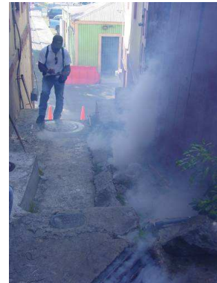
Smoke Testing to Locate Deteriorating Sewer Line, St. Thomas
