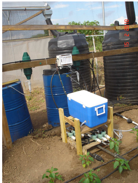
Pump, Injectors and Valves in Solar Powered System
