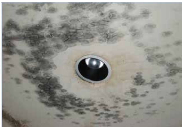
Ceiling covered with mold
