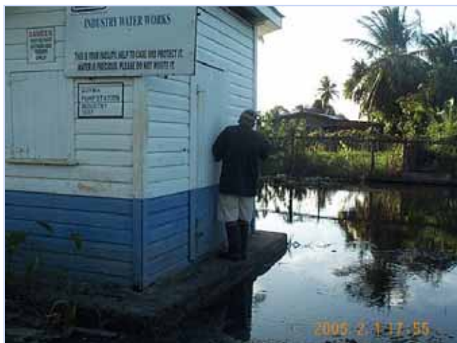
One of the GWI's pump station under water
