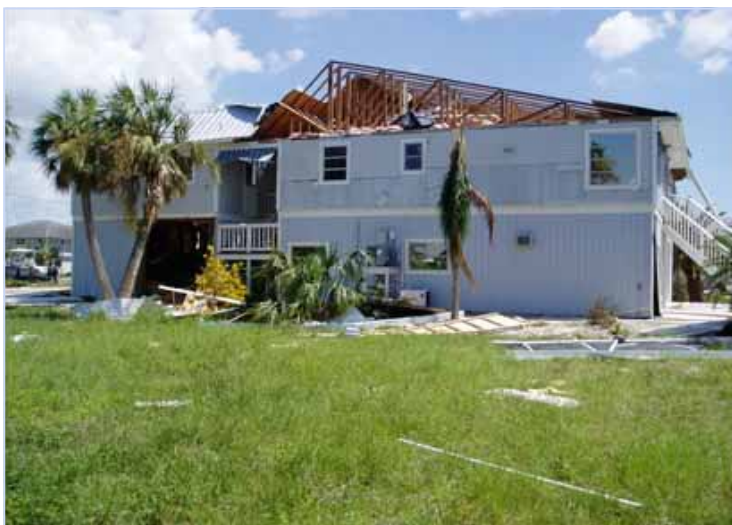
Severe roof damage to a home
